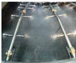
Spray bars with nozzles providing a pressure-less, balanced and efficient water cooling
